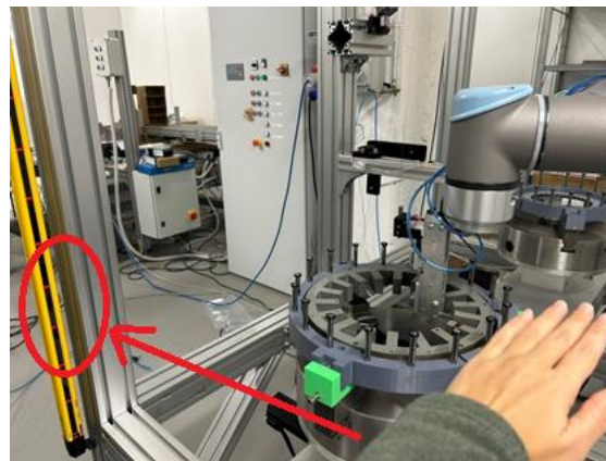
Figure 8: ICPE winding safety light curtain – red mode: entering the robot space
